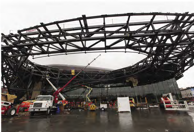
This page The center's cantilevered main entrance canopy is supported by two 12-foot-6-inch-deep primary trusses joined with diagonals, creating boxed trusses that tie back into the superstructure's columns. Facing Design architect SHoP's diagrams of the 110-foot-wide, 60-foot-deep entrance oculus (top) and panel system (bottom).
