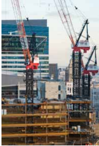
Far left The northeast elevation. Left The west elevation. Below The building's L-shaped site, as seen from above. Facing Steel framing allows the building to have a unique cantilevered shape, creating column-free corners and office floors adaptable to a range of uses.
