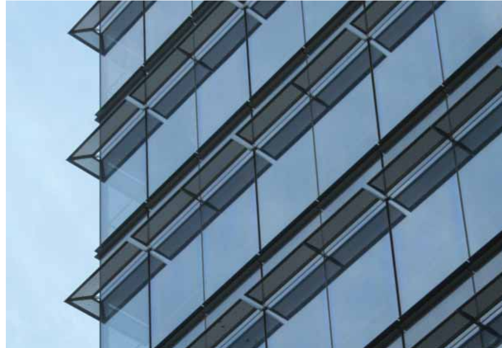
Above Perforated aluminum sunscreens attached to the unitized curtain wall reduce the building’s energy consumption. Left The tower’s shape maintains lines of sight on 42 nd Street.
