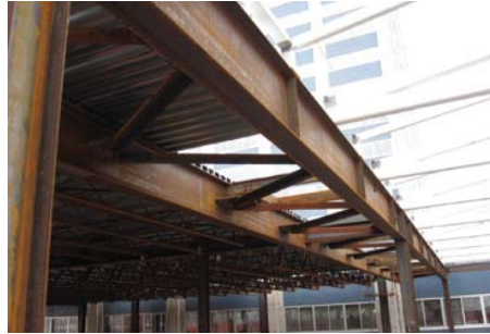
Clockwise from top Atrium HSS framing; the horizontal roof truss takes lateral loads from the main pavilion frames and transfers them to frames at the atrium perimeter; web penetrations; the atrium truss meets the mural wall truss.
