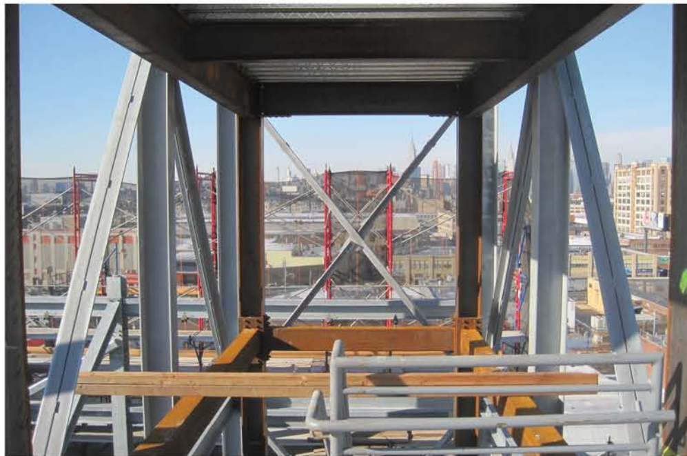
Top Steel framing of the training center's new multipurpose level. Above Structural steel framing for the rooftop beacon tower. Facing top A steel canopy shades outdoor space on the center's rooftop. Facing bottom The new multipurpose space faces views of Manhattan.
